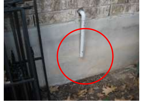
TPR discharge pipe to high
