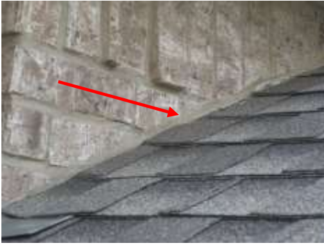
Counter flashing missing
