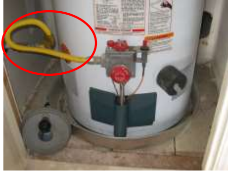
Drip leg missing
