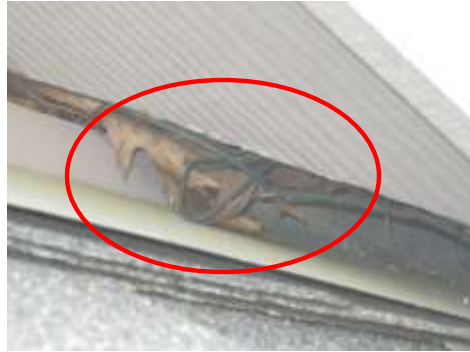
Previous signs of repair
